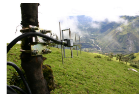
(c) Yagi antenna oriented towards observatory.
